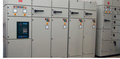
Elektrik pano üretimi Electricity board production
