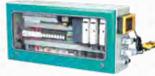
● Elektrik Panosu Electric Panel
