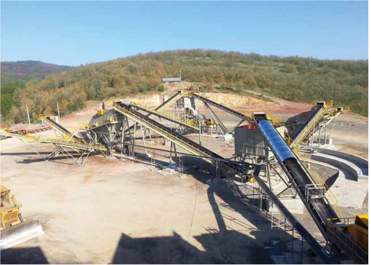
450-500 T/S Kapasiteli Kırma Eleme Tesisi Bulgaristan 450-500 TPH Capacity Crushing Screening Plant Bulgaria
