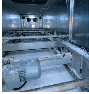
ICE STORAGE SYSTEM
