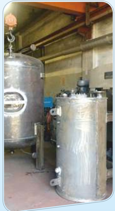
Thermal Oil Tank
