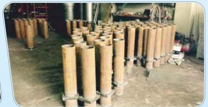
Demineralised Water Tank Anchorage
