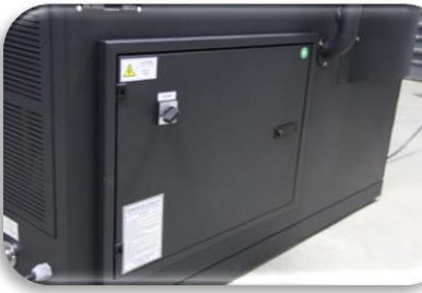
Concealed Electrical Panel
