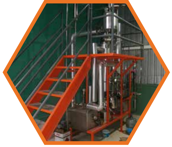
Thin Film Pilot Tesisi Thin Film Pilot Plant
