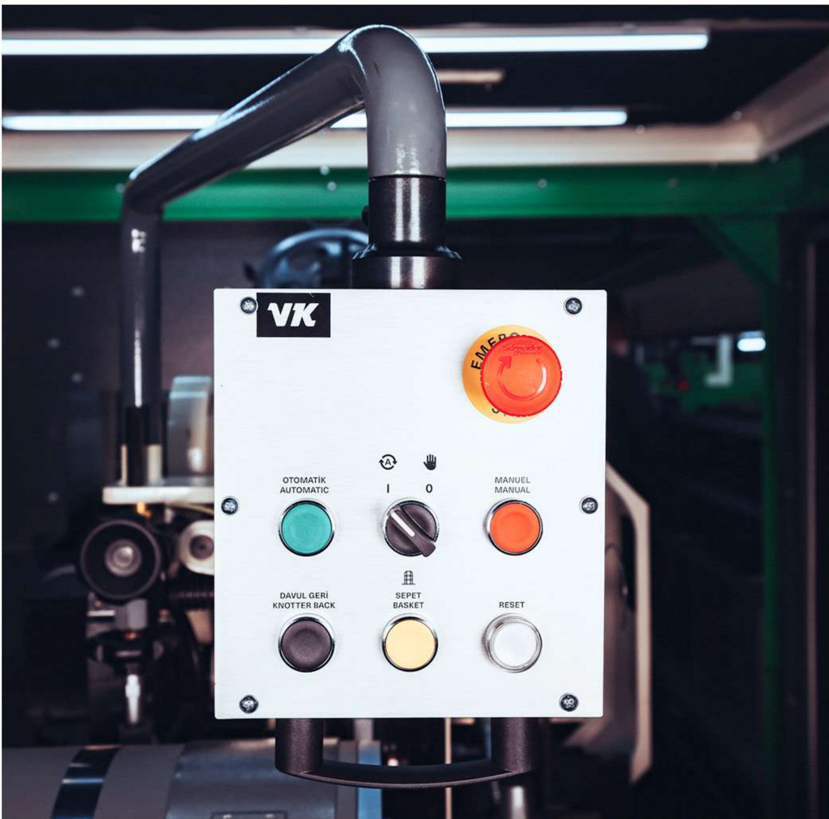
— Coiling Control Panel
