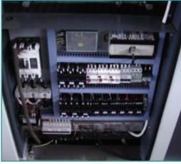
Electrik kontrol kabini Electrical control cabinet
