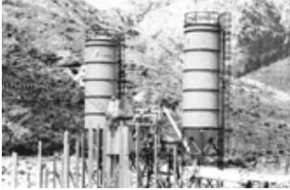
Beton Santrali Conc. Batching Plant
